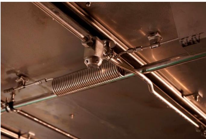
Caption: Extinguishing device as part of the safety concept for testing battery packs [Credit: ASAP Group]
